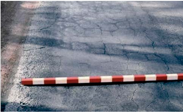
Figure 18. Fatigue cracking (= alligator cracking) in an asphalt mixture (from [45]).
