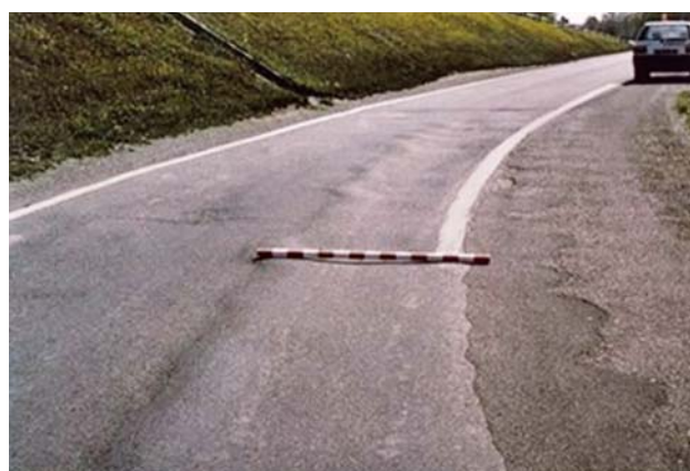
Figure 15. Rutting in an asphalt mixture (from [45]).
